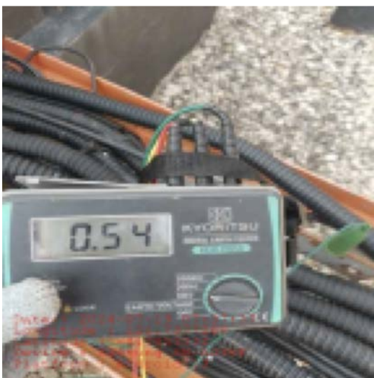
BAR GROUNDING TOWER
