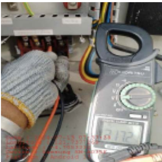
PENGECEKAN PHASE VOLTAGE
