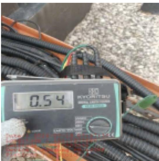
BAR GROUNDING TOWER
