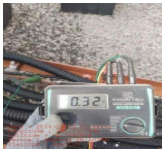
IGB / INDOOR SHELTER
